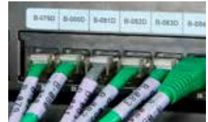
Patch Panel Labels
